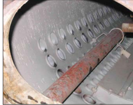
1st Inspection Dec. 04 (Close Up)
