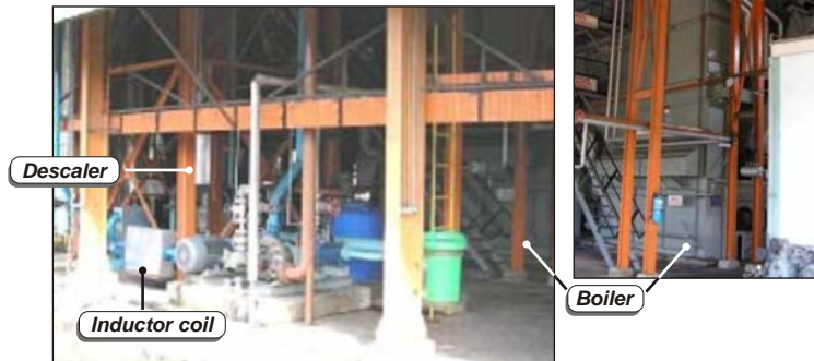
35 Tons Water Tube Boiler External View
